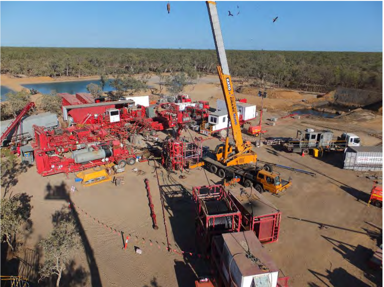
Figure 4 Hydraulic fracturing operation at the Egilabria-2 well pad in the Isa GBA region
